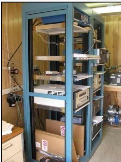
Air Quality Monitoring Equipment
