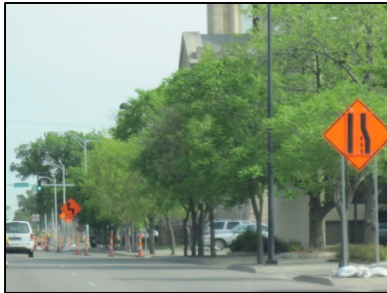
Work Zone Signs
