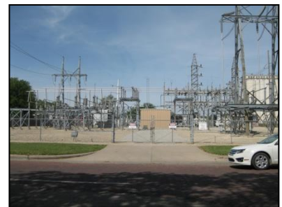
Power Plant Substation
